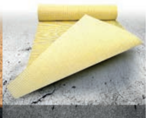
Installation on cracked floor screed
